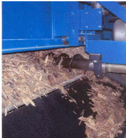
Merrimack Valley High School recently constructed this wood chip biomass boiler to heat its physical plant.
